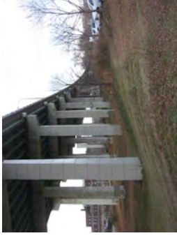
5. View west along the slope of the cut on the south side of the west parking lot.
